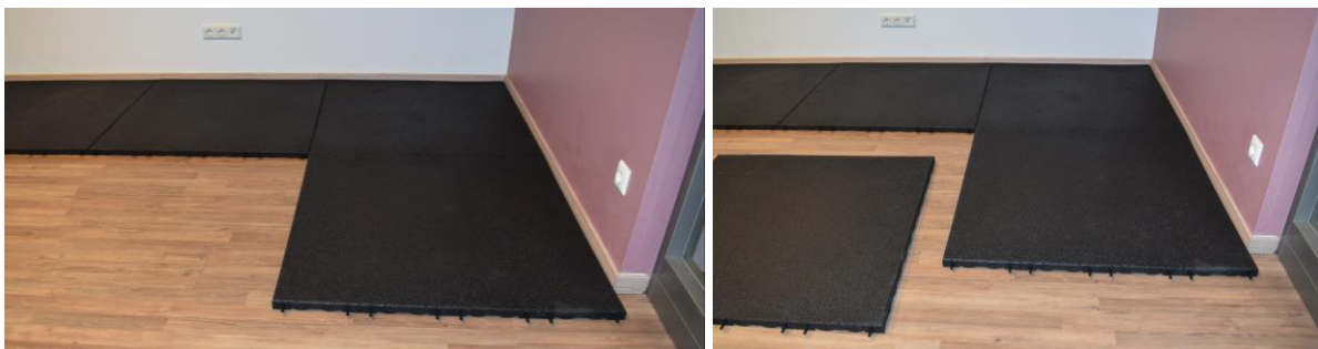
Start the second row of the tiles in the same way and continue; place the tiles next to each other
