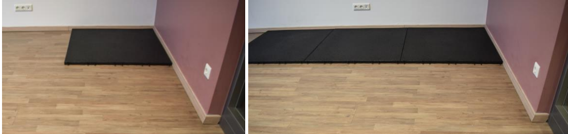
Installation of the tiles along a wall with the connector pins towards the next row
