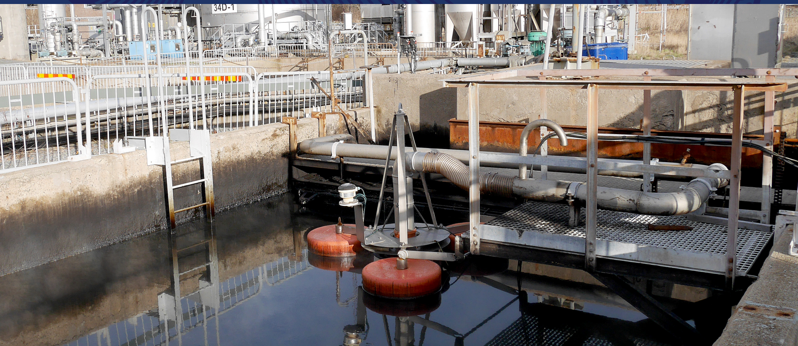
A SurfCleaner SCO 8000 operating in an API basin.
